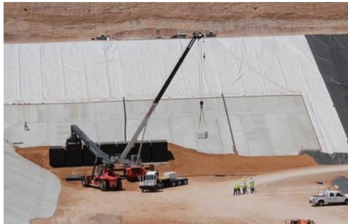
Figure D-5. Wastes Being Loaded into Modular Concrete Canisters at the Waste Control Specialists Disposal Cell
