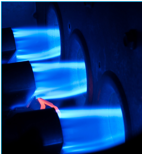
Figure 6.11. Heating chamber inside a gas furnace.
