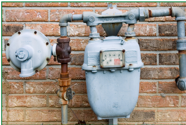
Figure 9.2. Natural gas meter.
