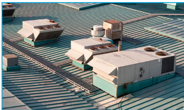
Figure 6.7. Example of several packaged rooftop units.
