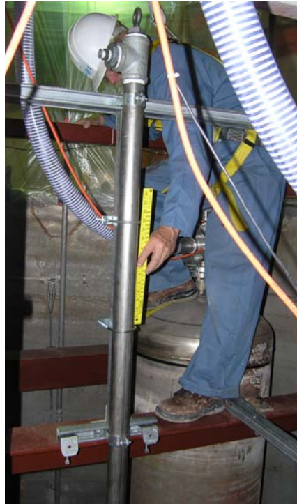
Figure 5.8. The Mount for the Accelerometer Mast
