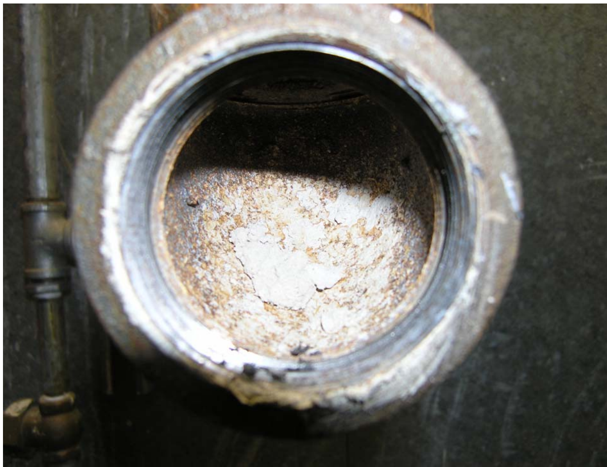
Figure B.1. Clay Deposit in 90° Elbow of the Air Line from PJM #5
