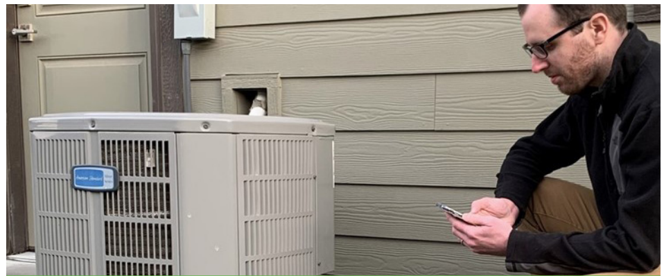
An example of HVAC Smart Diagnostic Tools
