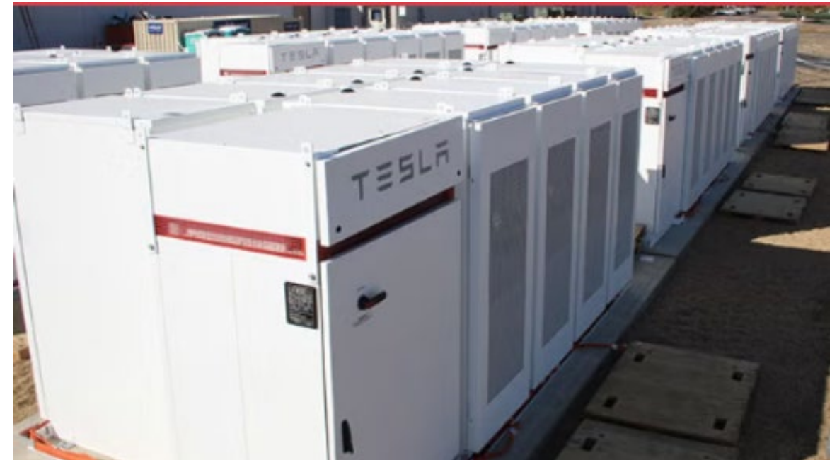
United Power Cooperative's Carbon Valley battery storage facility
