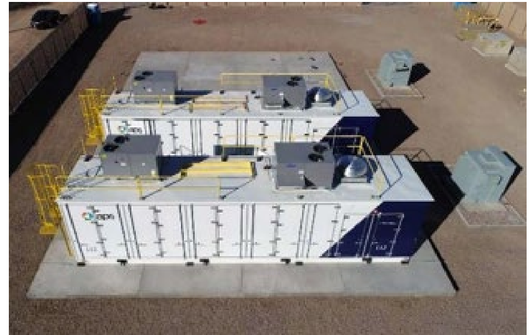
Overhead view of the Punkin Center BESS facility
