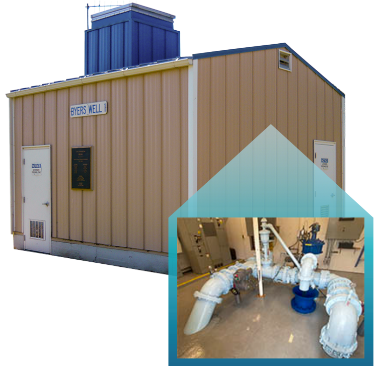
Well #14 Hydropower Installation. Photo credit City of Pendleton, Oregon
