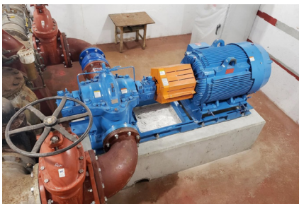
10 kW pump as turbine installed at the Narrows Road Water Treatment Plant in Fitchburg, Massachusetts
