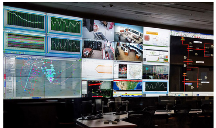
The Electricity Infrastructure Operations Center at PNNL is one of several key facilities that underpins the Modeling and Tools core competency.
