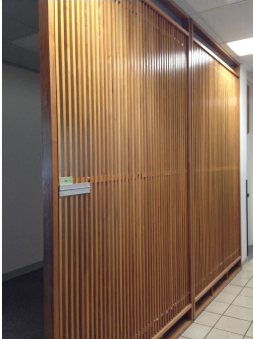
Figure 11. Decorative Vertical Wooden Screens Separate the Reception/Secretary Offices from Hallways in Building 520
