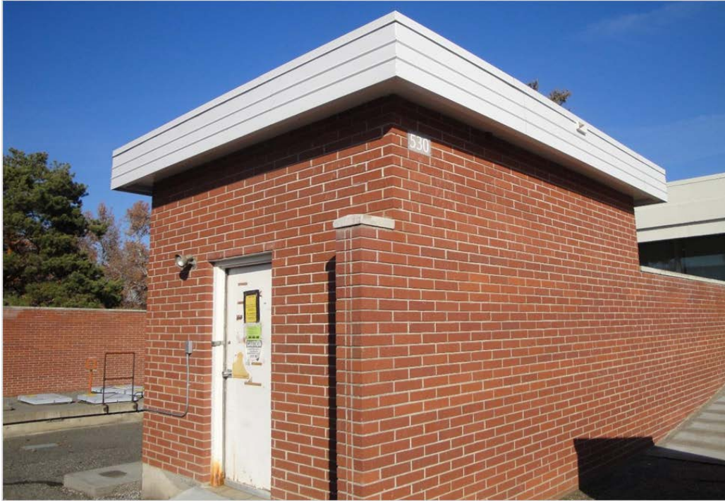
Figure 5. RTL 530 Southwest Corner (Harvey et al. 2015)
