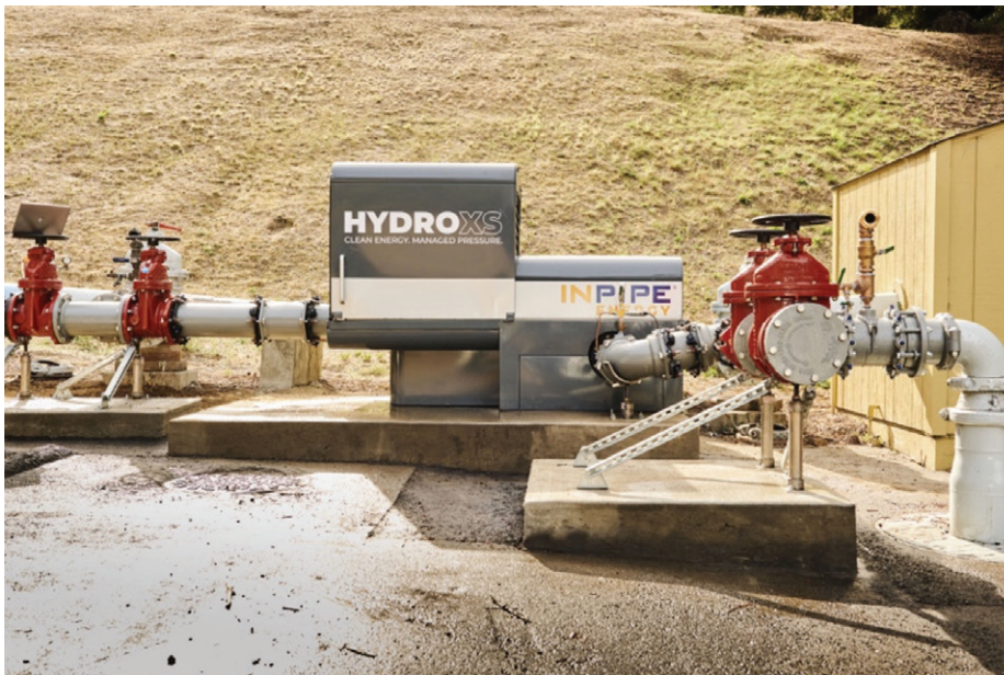
HydroXS system installed at one of the East Bay Municipal Utility District’s pumping stations. (Photo Credit: InPipe Energy)
