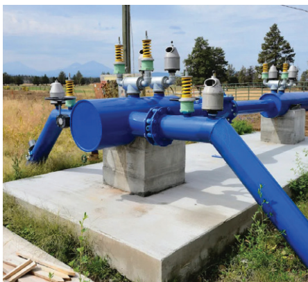
Farm turnouts where PRVs are installed. Photo credit: Energy Trust of Oregon
