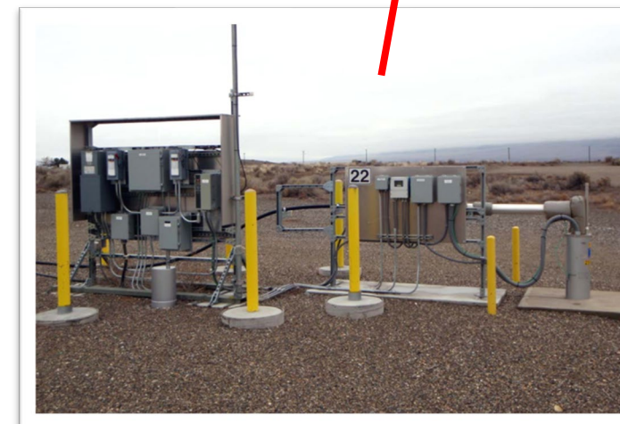
Pump-and-treat extraction well (adapted from PNNL-24741)
