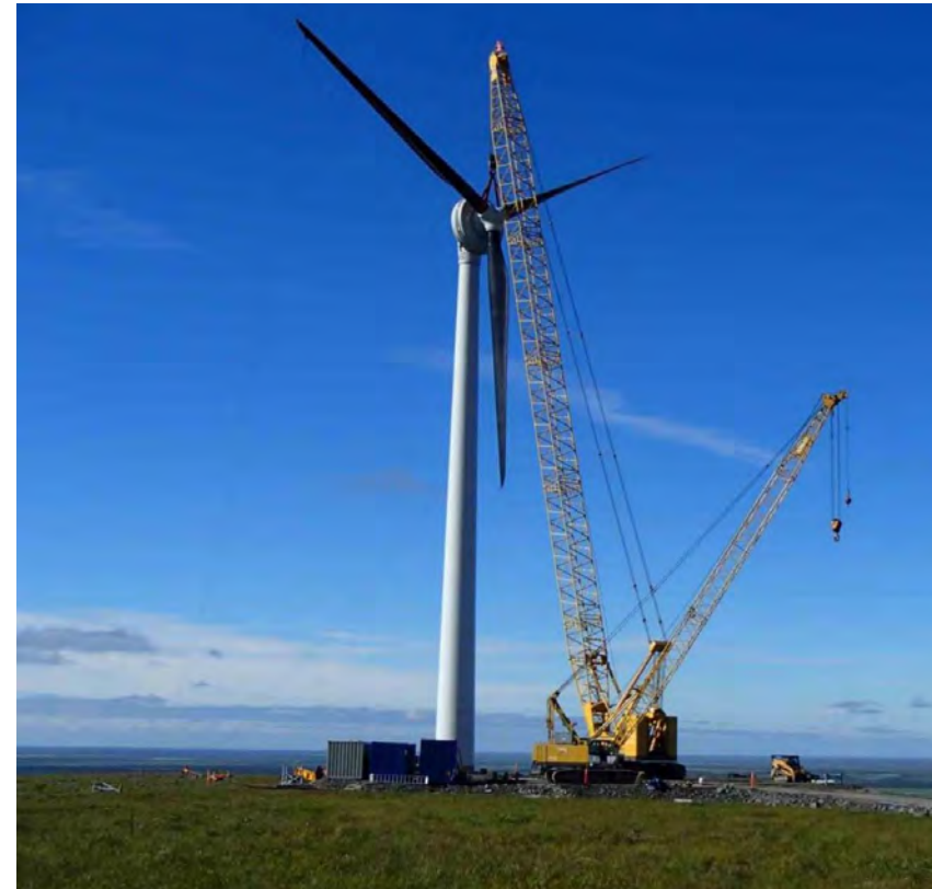
The St. Mary's Community Wind Turbine, Alaska (Photo: US Department of Energy)
