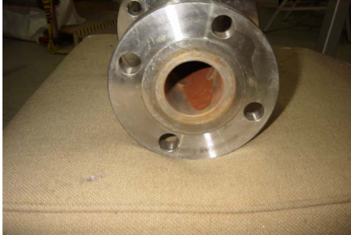
Inlet to Pipe Reducer, View F
