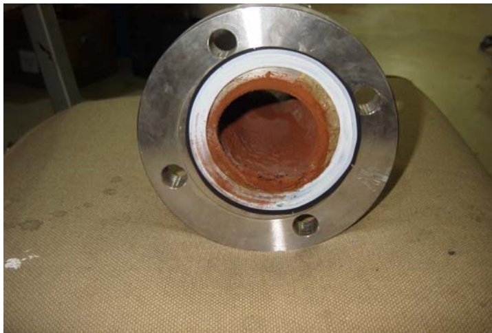
Outlet of Pipe Reducer, View G
