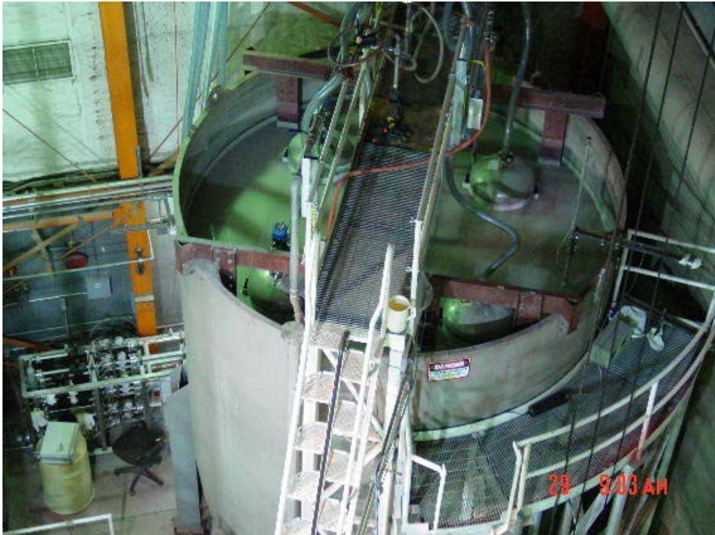
Figure 2.3. Photograph of the Top View of the LTTS Showing the Structure Used to Support the PJMs
