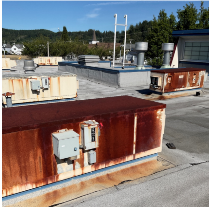
Figure 2.1. Rooftop HVAC units at Central Elementary
