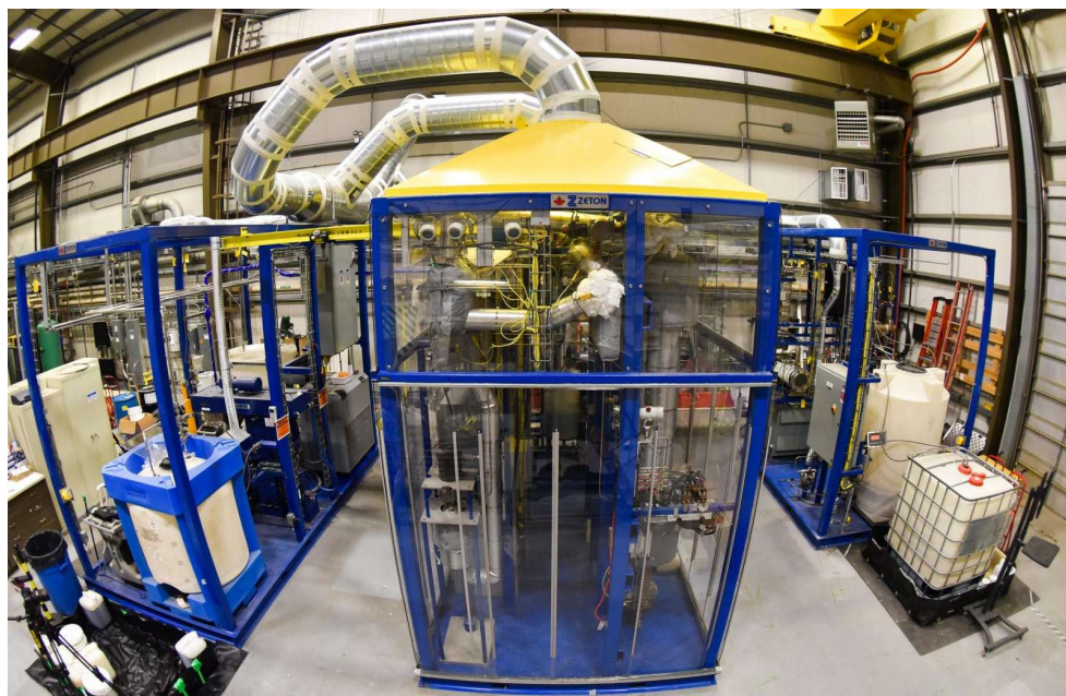
Figure 2. Photo of the MHTLS at PNNL.
