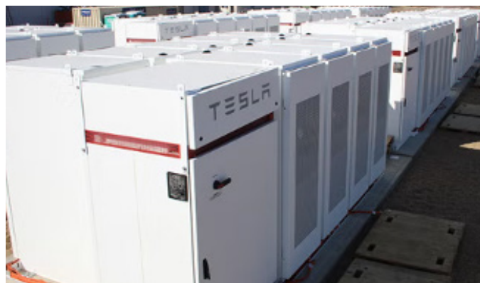
Figure 1. United Power Cooperative’s Carbon valley battery storage facility. 2
