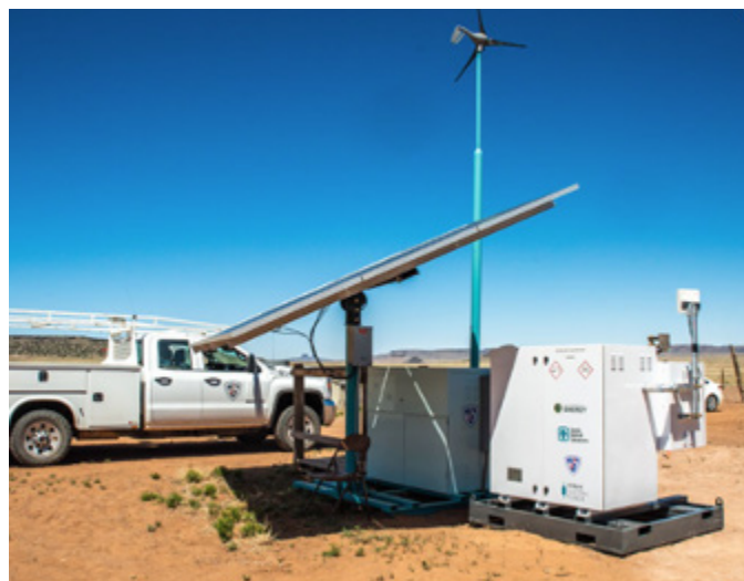
Figure 4. Installed BESS and solar panels in Dilkon, Arizona. 6
