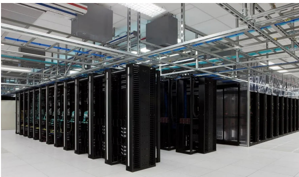
Figure 12: Representative Data Hall [23]. This Facility is Rated for Tens of Megawatts, Tier IV Reliability, and LEED Gold Efficiency.
