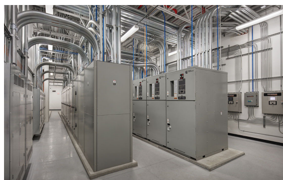
Figure 11: Electrical Room for Medium-Sized Data Center [22].
