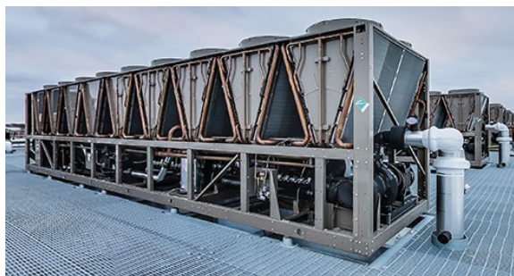
Figure 15: Large Rooftop Chiller Unit for Data Center [21].
