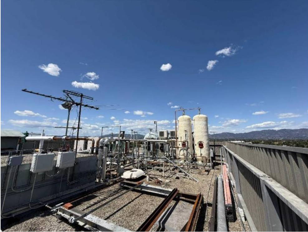
Figure 5 Full CHPWH system at Casa Panorama with M&V panels at left
