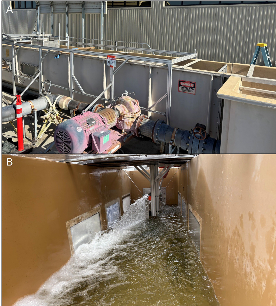
Figure 2-1. (A) Side view of the PNNL shear tank showing the pump motor, and (B) a view from the interior of the shear tank facing the jet nozzle.
