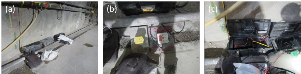
Figure 9. Photographs showing the (a) co-located geophone and accelerometer installations; (b) an example geophone and accelerometer; and (c) an example digitizer and the power source. Photos by K. Chojnicki.
