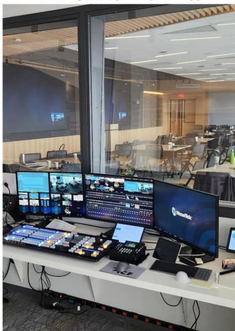
A. ICF Meeting Facility for Hybrid Support
