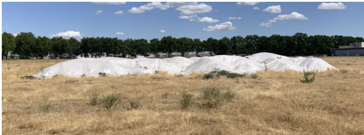
Figure 13. Recent photo of the stored stockpiled soil removed from the Tank Pit during excavation.
