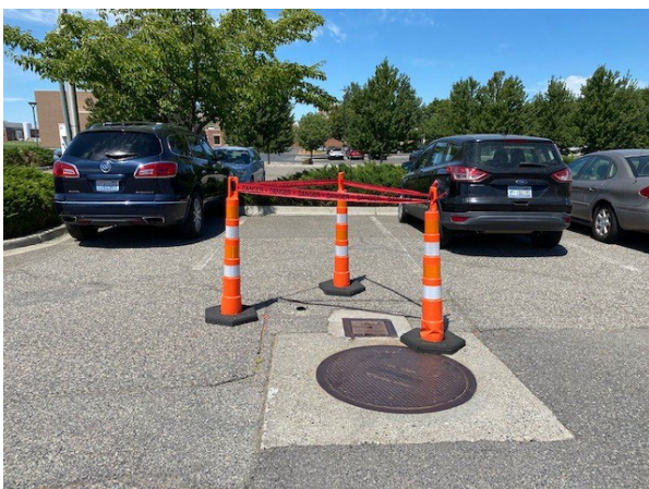
Figure 3. The location in the parking lot where the tank and tank access covers re located, facing north, taken July 2022.
