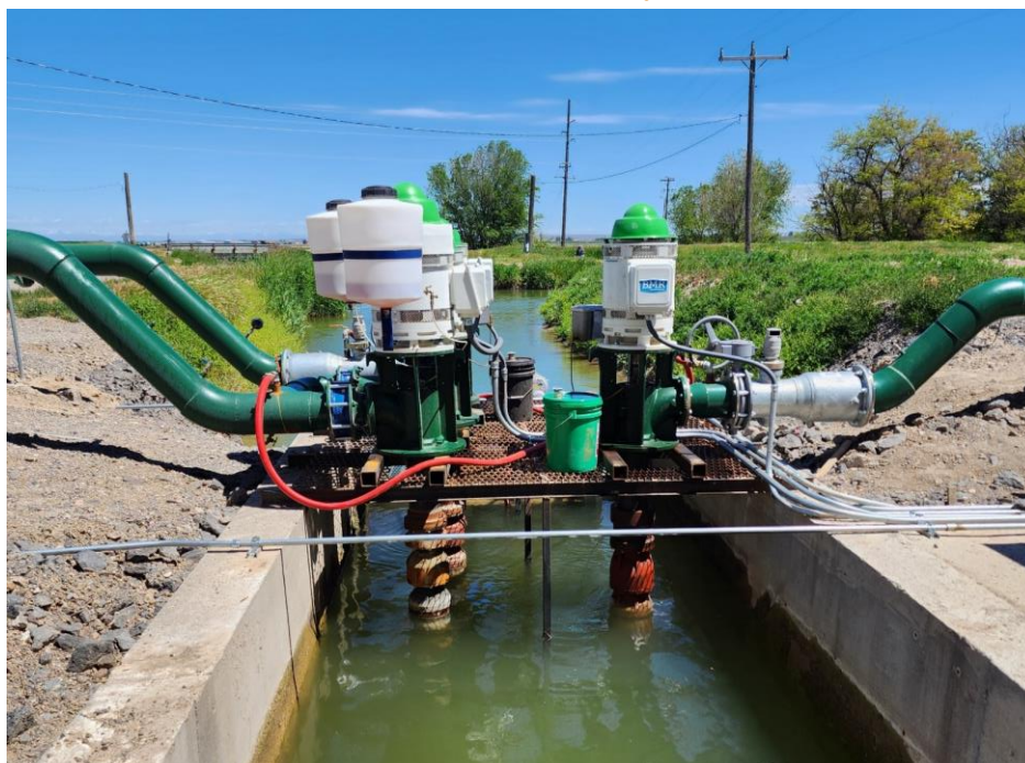
Figure 10. An array of modern on-farm pumps, powered with variable frequency drives, on a lateral in the North Side Canal Company near Jerome, Idaho. Photo credit: Camilo Jose Bastidas Pacheco | Idaho National Laboratory.
