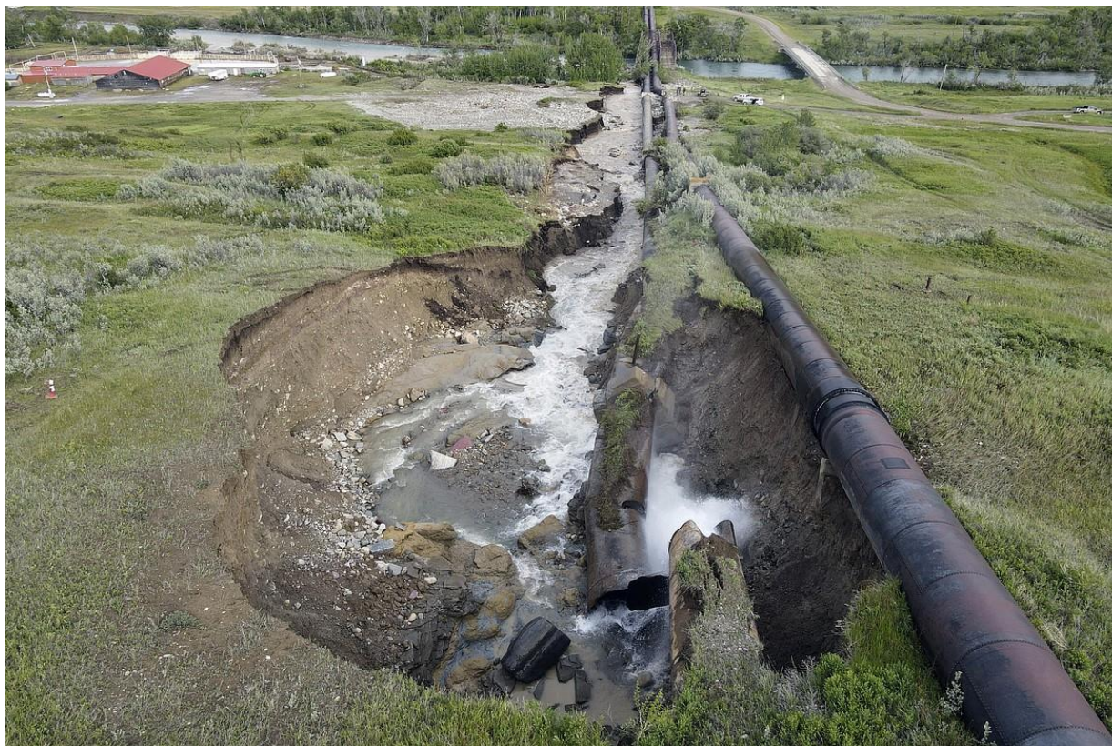
Figure 6. The St. Mary siphon failure resulted in erosion and flooding. According to the Milk River Joint Board of Control, the two pipes are each 7.5 feet in diameter and were transporting approximately 600 cubic feet of water per second. (Photo credit: Bureau of Reclamation)
