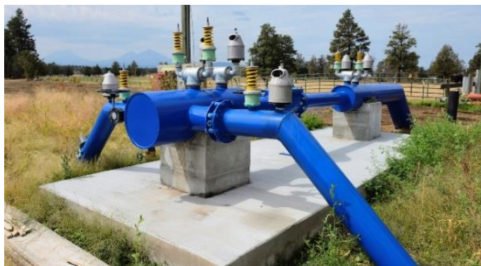
Figure 11. Piped delivery point where surplus pressure could produce hydropower. (Photo credit: Energy Trust of Oregon)
