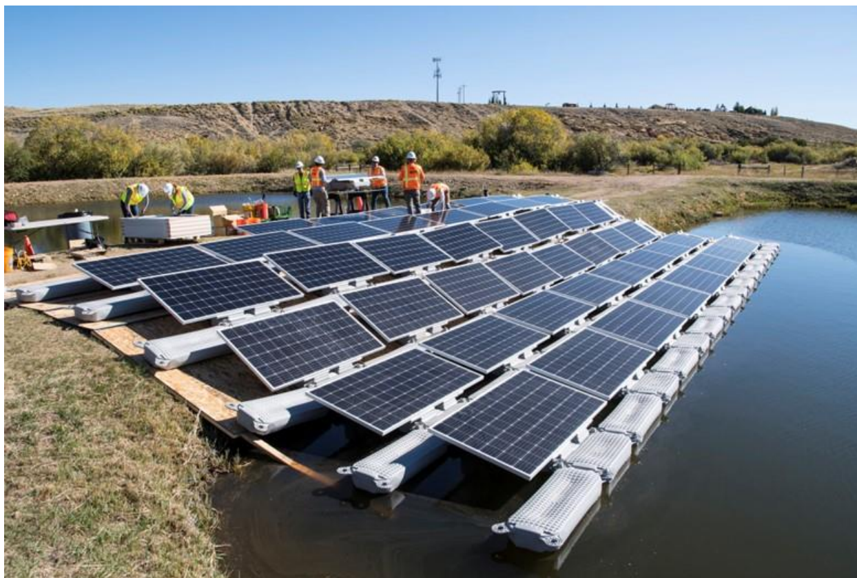
Figure19. Floating solar demonstration project (Image: National Renewable Energy Laboratory). 1
