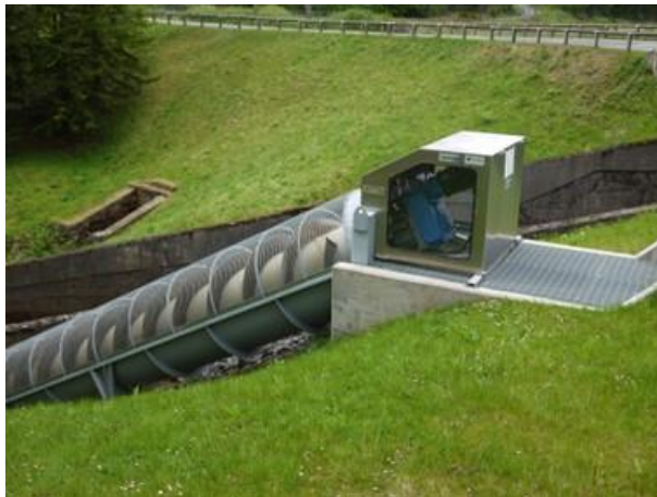
Figure 12. A small-scale Archimedes screw generator unit in the United Kingdom (Image: Christopher Down). 1
