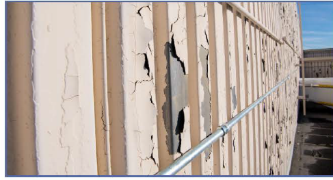
RPL's siding before replacement. Photo by Andrea Starr | Pacific Northwest National Laboratory
