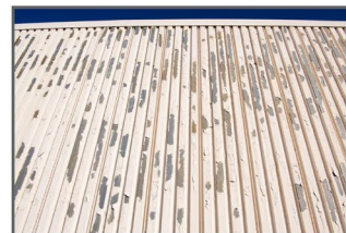
RPL's siding before replacement. Photo by Andrea Starr | Pacific Northwest National Laboratory
