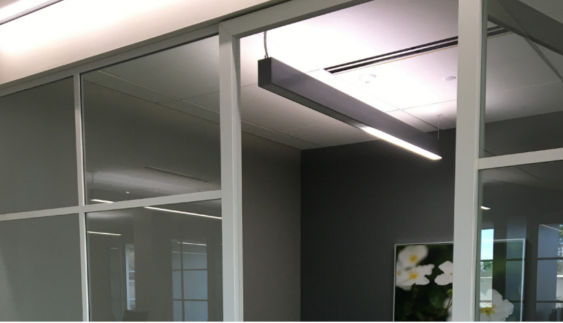
Figure 7: An 8-ft-long direct/indirect luminaire in a conversation room, with one half of the downlight responding incorrectly. Photo: SimTigrate Design Lab.
