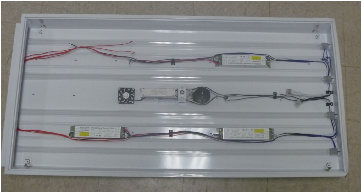
Figure 32. Two views of LPM-22-07A. Image (a) shows damage to corners of housings typical of all units received. Image (b) shows the internal ballast compartment, where one of the four 1-lamp ballasts was missing. Notably, the internal fan for this product is visible left of center.
