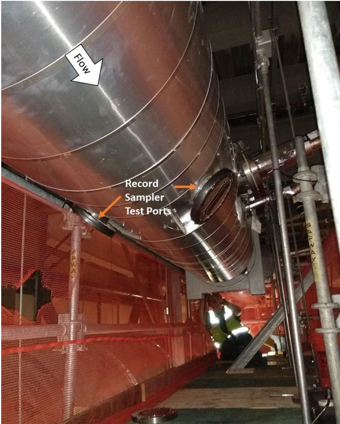
Figure 4. LAW LV-S3 Stack. The pair of ports to characterize the RS port location is visible in the foreground (near the center of the image) while the ports to characterize the CAM is in the background, at the location of the Bison staff member. The stack is positioned near the center of the L-0320 Stack Monitoring Room, and the photograph is nominally pointed to the north. Stack flow is from the foreground (south) to background (north).
