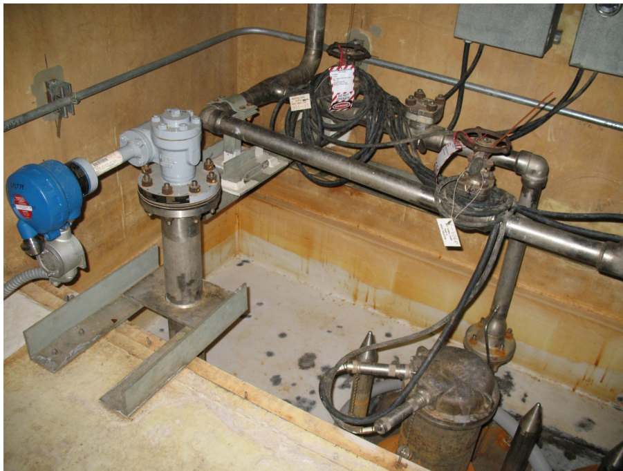
Figure 3-11 Sump well and recirculation system. (Generic photo.)
