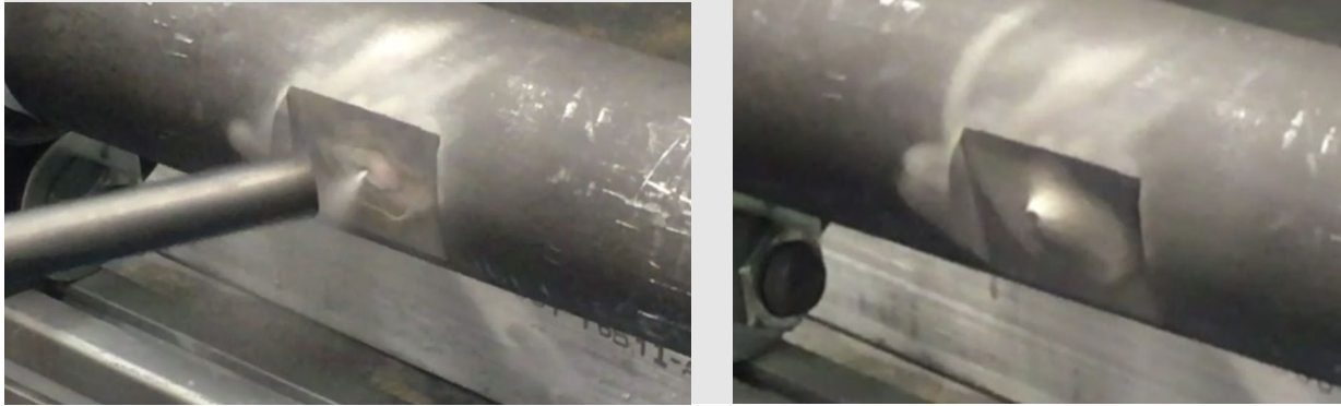
Figure 3-8 Repair of active leak using CS by VRC Metal Systems. Left: water leak; right: final repair. Pressure of the pipe was ~100 psi during and 1,000 psi after the repair (Ross and Alabi 2019).
