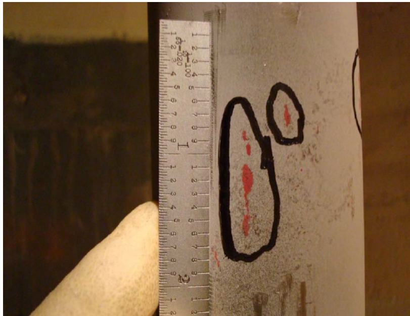
Figure 3-6 Example of CISCC under a pipe hanger in an ECCS piping section. The pipe hanger provides a concentrating mechanism for chloride entrapment, producing cracking in locations that are not accessible for visual inspection. (PNNL presentation on CISCC)
