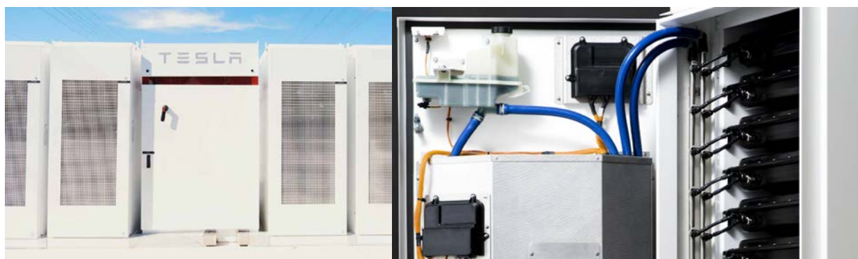
Figure 3.3. Tesla Powerpack 2 Lithium-Ion Energy Storage System – Exterior and Interior
