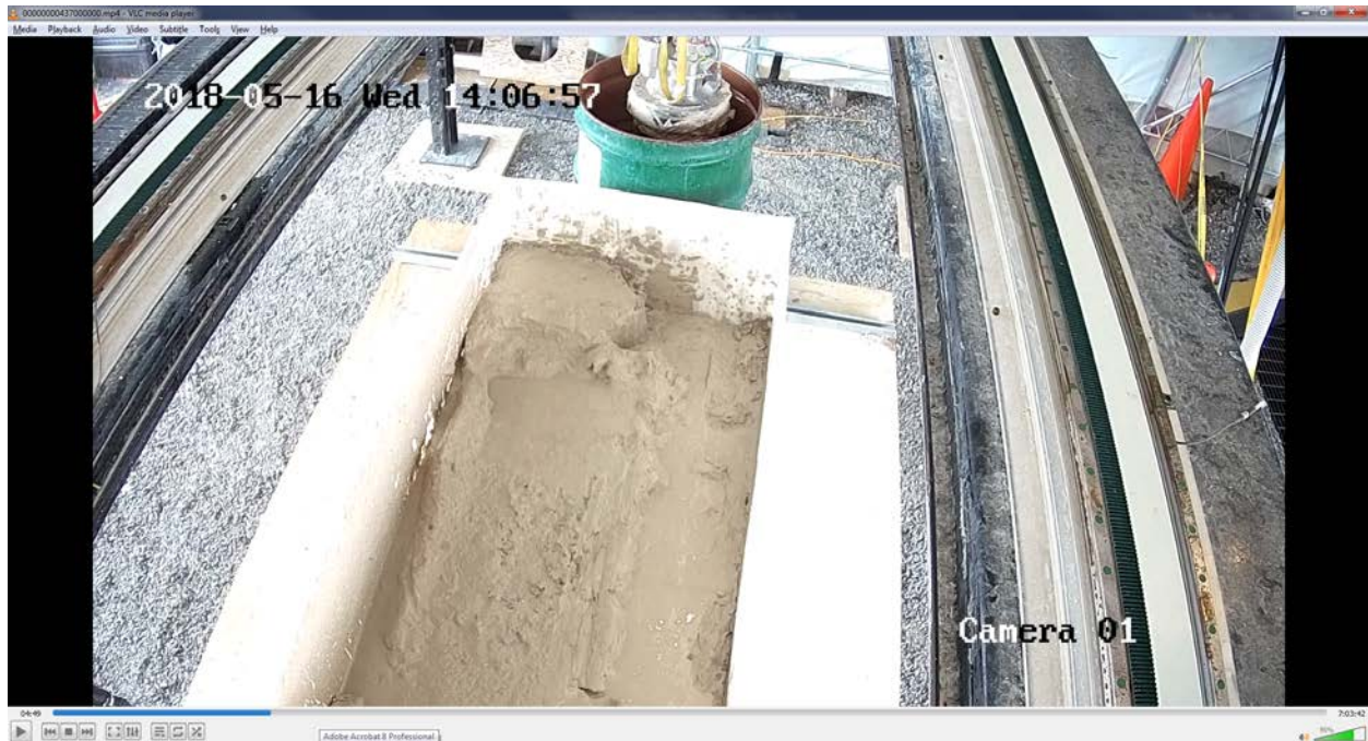
Figure TS21 – Setting HWEE pressure (1000 psi) in Capture Tank
