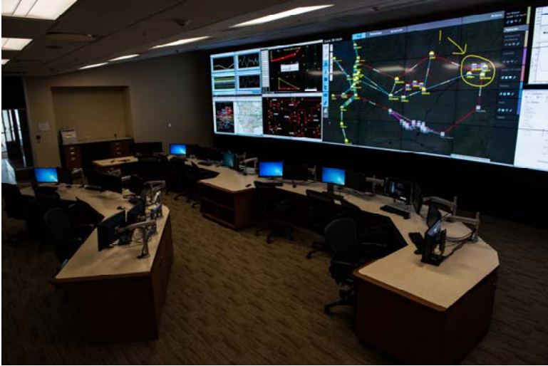
Figure 3. EIOC West Control Room
