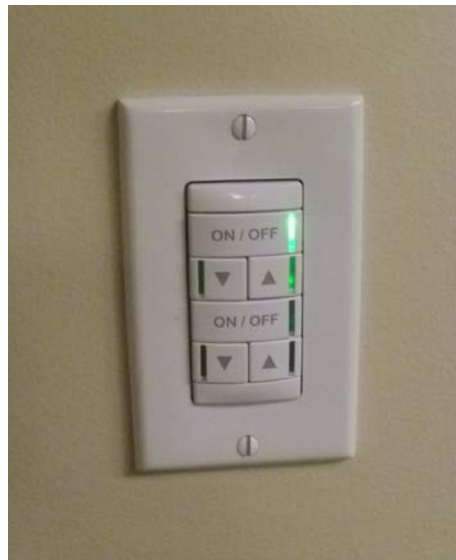
Figure 8. Wall control in large conference room, with separate raise/lower functions for the Acuity Brands Winona® Trilia™ pendants and the Birot Zhen pendants. Photo: PNNL.
