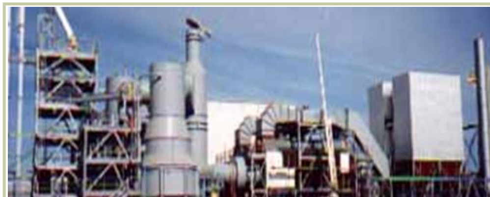
Fig. 5. Dual reactor air fed gasifier of the general design as that depicted in Fig 4. (From left to right: bucket elevator for RDF feed, gasifier reactor(s), combustion tube, heat recovery boiler, baghouse and stack.)
