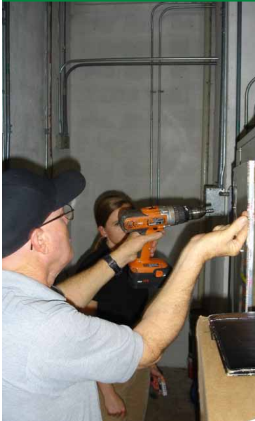
Companies may need to provide electricians or other staff to facilitate the audit.
