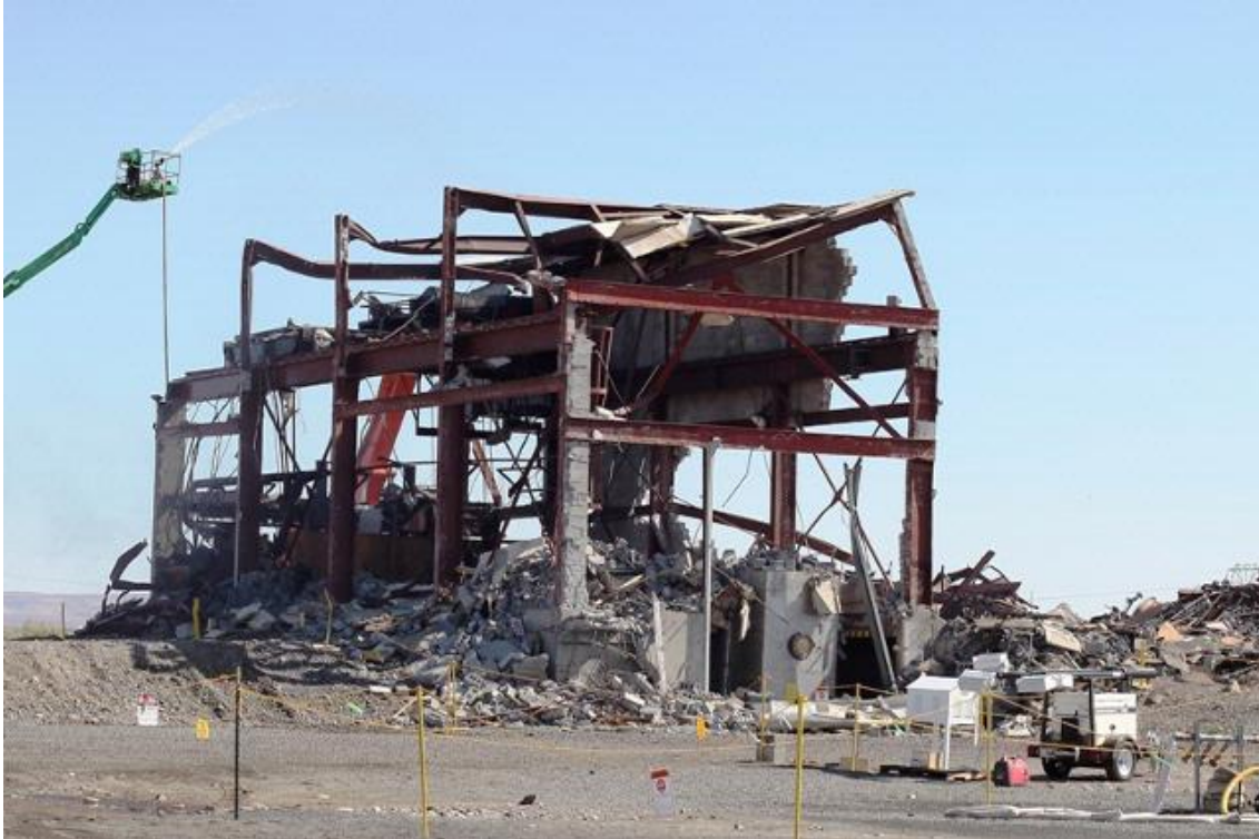
Figure A.5. Assumed Interim Demolition Conditions: Roof and Walls Rubblized Prior to Shearing of Steel Framework (212-R building used as example)
