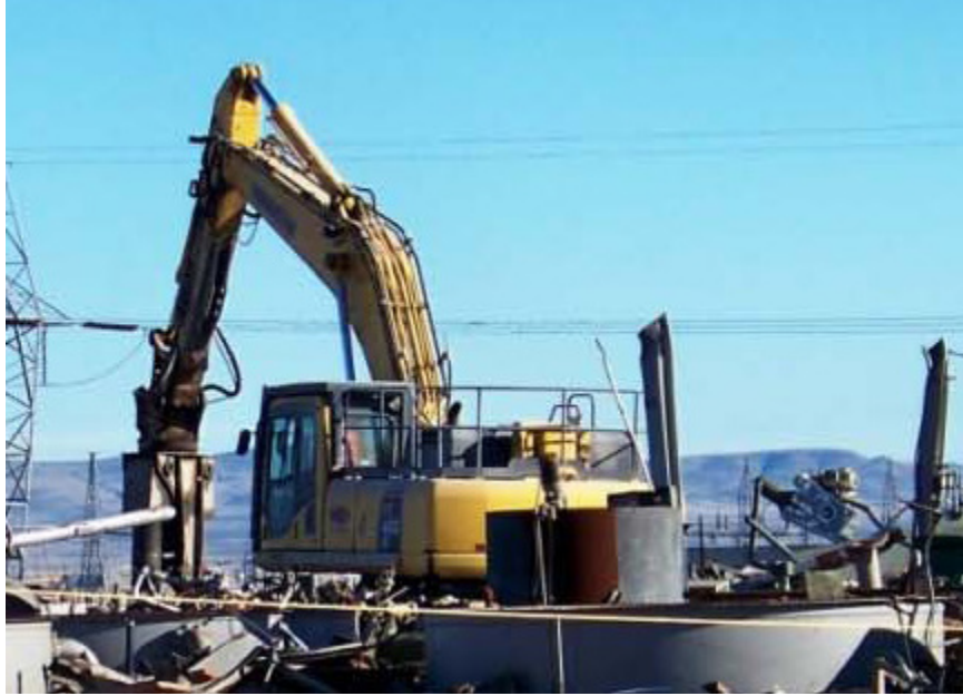
Figure D.4. A Multi-processor Size-reducing Large Pieces of Equipment
