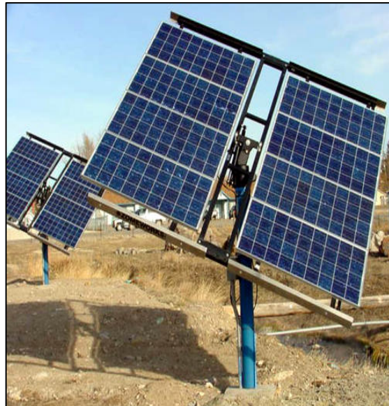
Figure E-1: Dual-Axis Tracking PV Array
