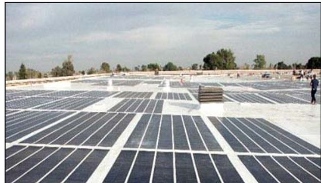
Figure E-2: Integrated PV on Rooftop
