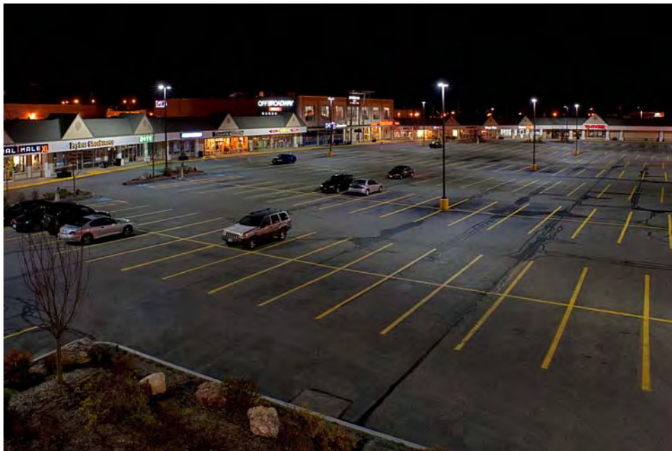
Figure 2.8. Parking Lot After Installation of LED Luminaires (Source: BetaLED)
