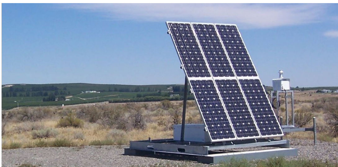
Figure 6.1. Example of 24-V Solar-Powered Particulate Sampling System (PNL-2)
