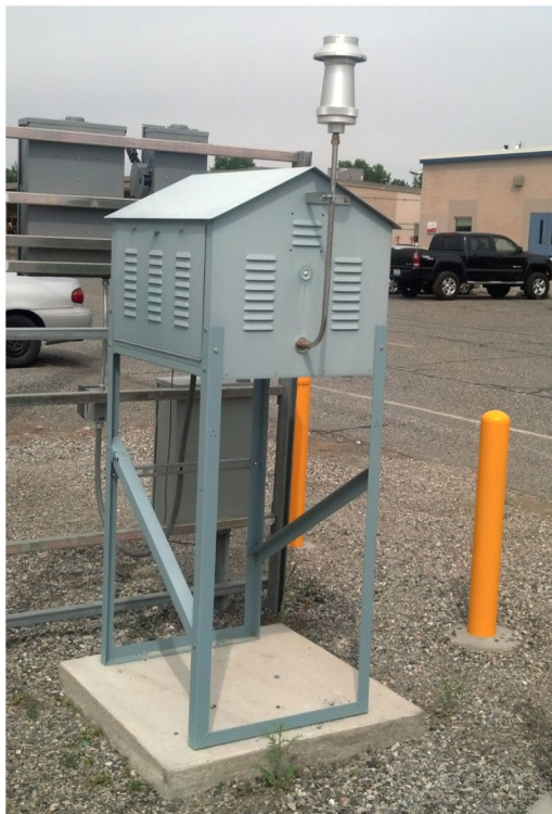
Figure 6.2. Example of 120-V AC-Powered Particulate Sampling System (PNL-4)
