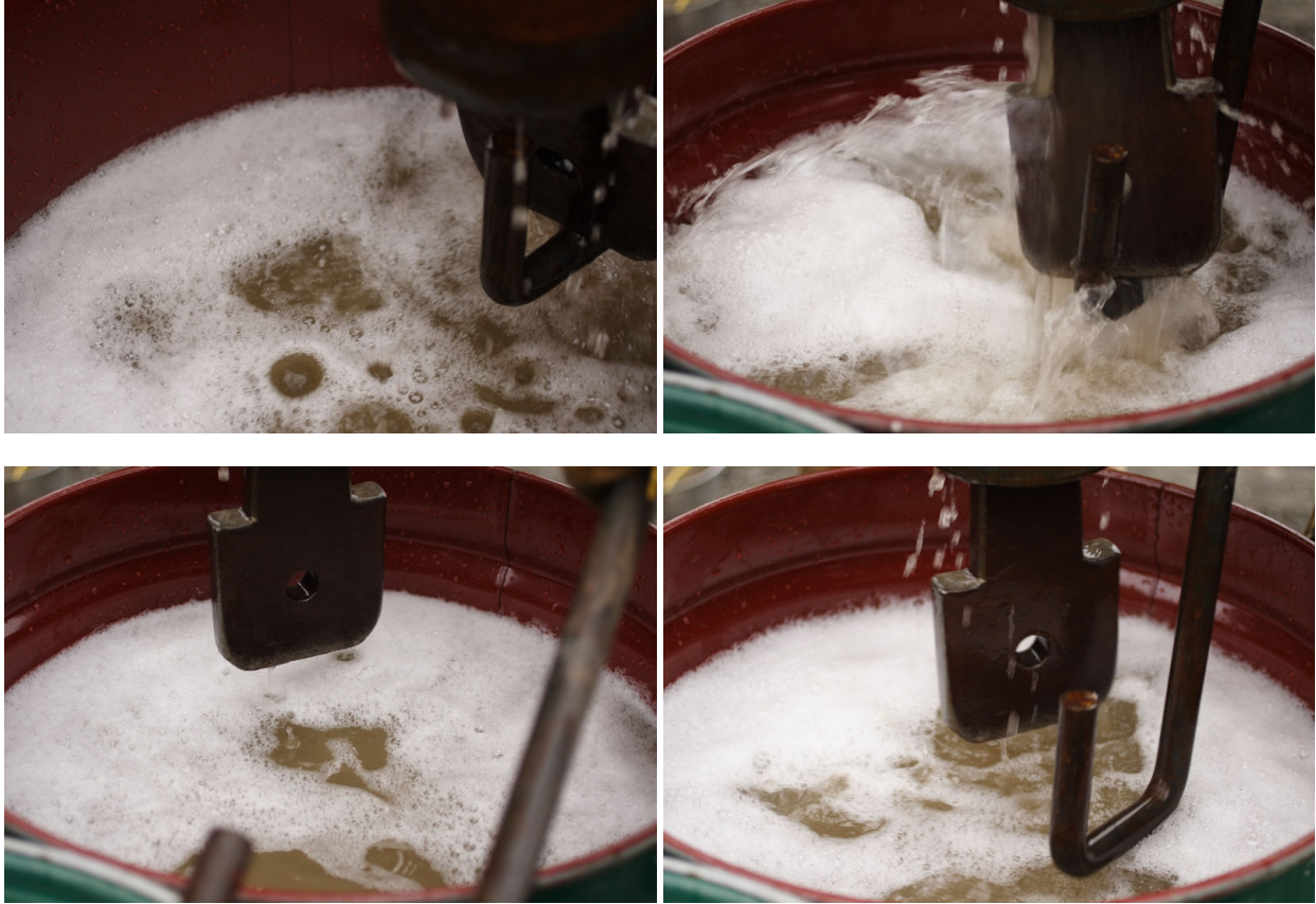
Figure C.3. Examples of the Unusual Foamy Water Observed During Drilling and Development of Monitoring Well 199-N-173
