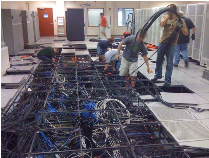
Before installing Phase 2 of Chinook, EMSL staff removed about 25 miles of communications cables that once passed data between the older supercomputer's nodes.
