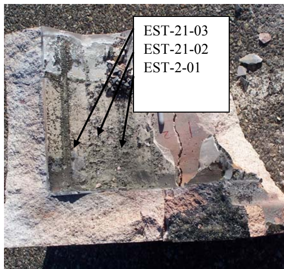
Figure 10. Corner Section of Tiled CRB with Base at the Bottom of the Photograph. Tiles have been removed from the Area Below and to the Right of the Pen. Note Large Crack Between the #1 and #2 was an Artifact of the Sampling Process.
