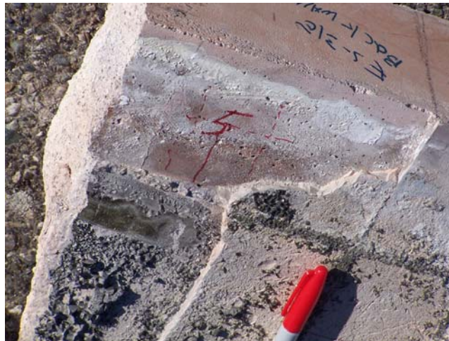
Figure 9. Upper Portions of CRB with Partial Tile Removal. Note Glass Penetration Behind Tile in Lower Left Hand Corner of Photograph. The “5” Indicates Where CRB Sample EST-21-05 Was Taken.
