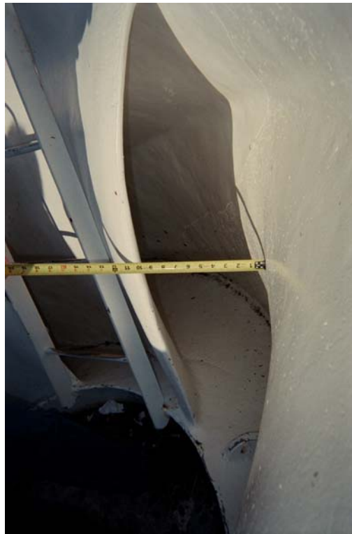
Figure 3.10. Measuring the width of the opening of the pump intake vanes. (The ladder shown in the picture is not a normal part of the runner.)
