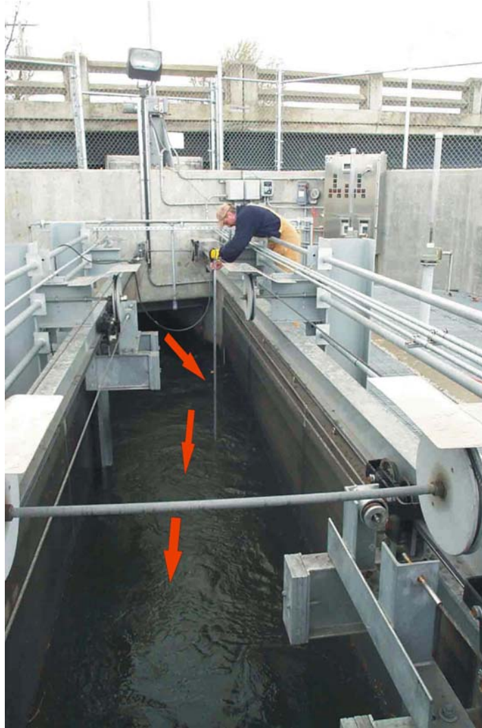
Figure 1.2. Nursery Bridge Fish Ladder Attraction Flow Screens. The red arrows show the direction of water flow.
