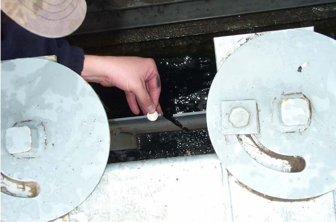
Figure 3.10. The Louvers at Nursery Bridge Fishway Attraction Water-System Screens Had a Gap the Size of a Nickle (Approximately 2.2 cm [0.875 in.]) Between Them when Fully Closed. This is a view from the top looking down at the water surface, with a quarter placed next to the gap in the louvers.
