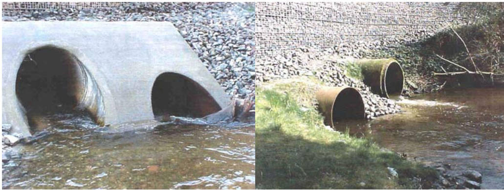
Figure 3. Dogfish Creek culvert inlet (left photo) and outlet (right photo), March 1999. Courtesy of Washington State Department of Transportation.
