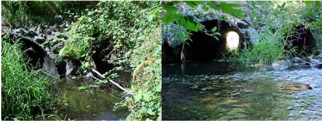
Figure 8. Snow/Andrews Creek convergence and culvert inlet (Andrews Creek, left photo) and outlet/convergence (right photo), August 2001.
