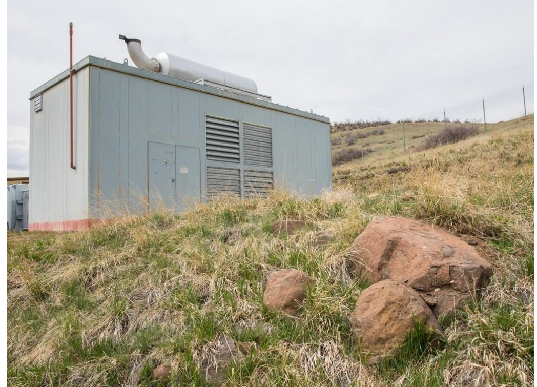
An emergency generator nicknamed “Big Buck” at NREL. (Photo by Werner Slocum/NREL)
